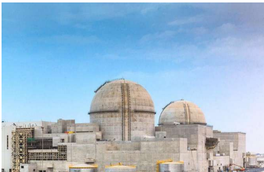
The UAE's Barakah nuclear power plant under construction in 2017. Photo by Wikimirati via Wikimedia Commons
