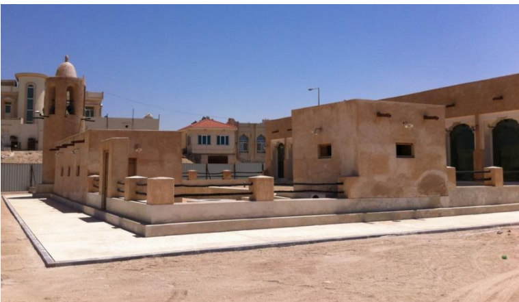
Figure 4. Al Dhakhira mosque, one of the recently completed conservative restoration and structural works. Source: Author.
